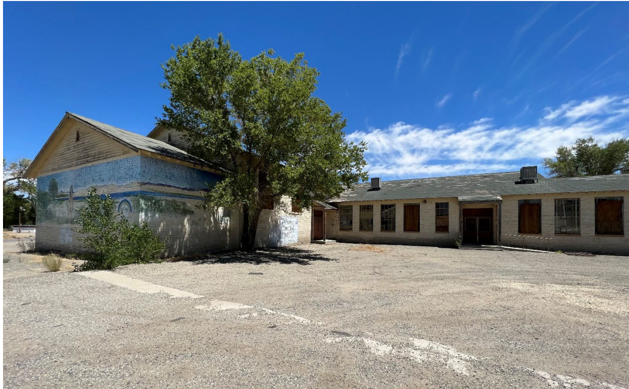
Figure 5. West side of the old school showing deteriorated roofing and paint.
