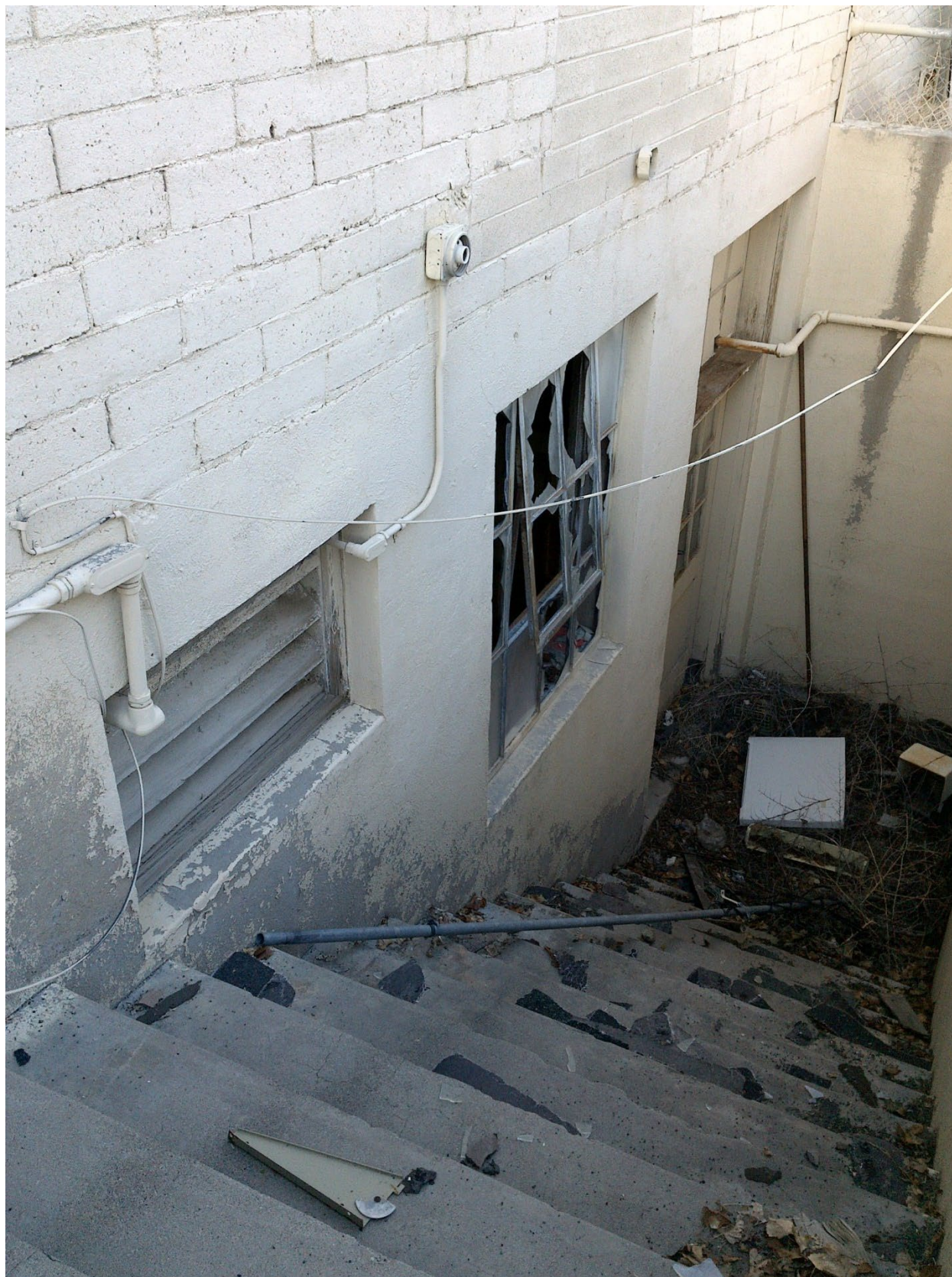
Figure 10. Basement access door and stairs located on the west side of the courtyard.
