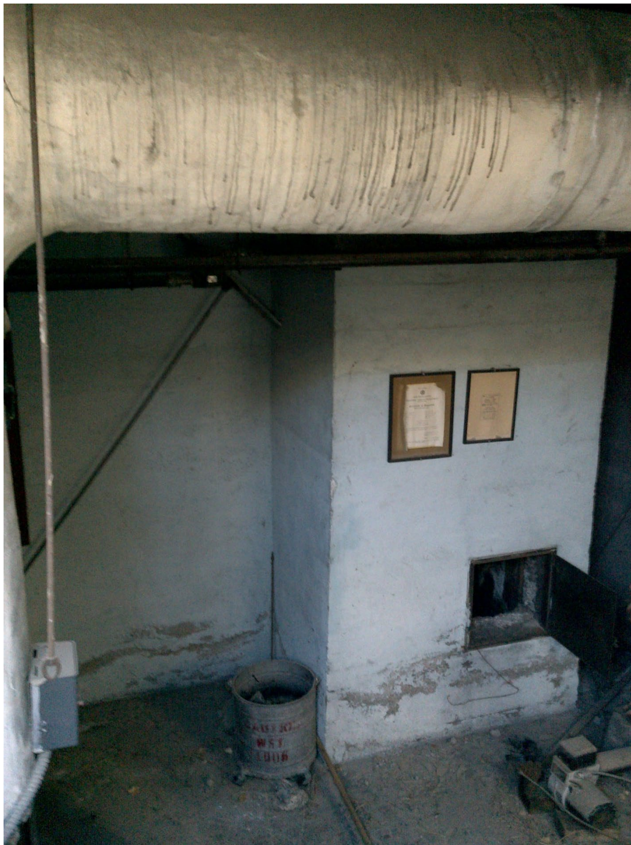
Figure 11. Basement boiler room accessed by the staircase and door in the previous figure.
