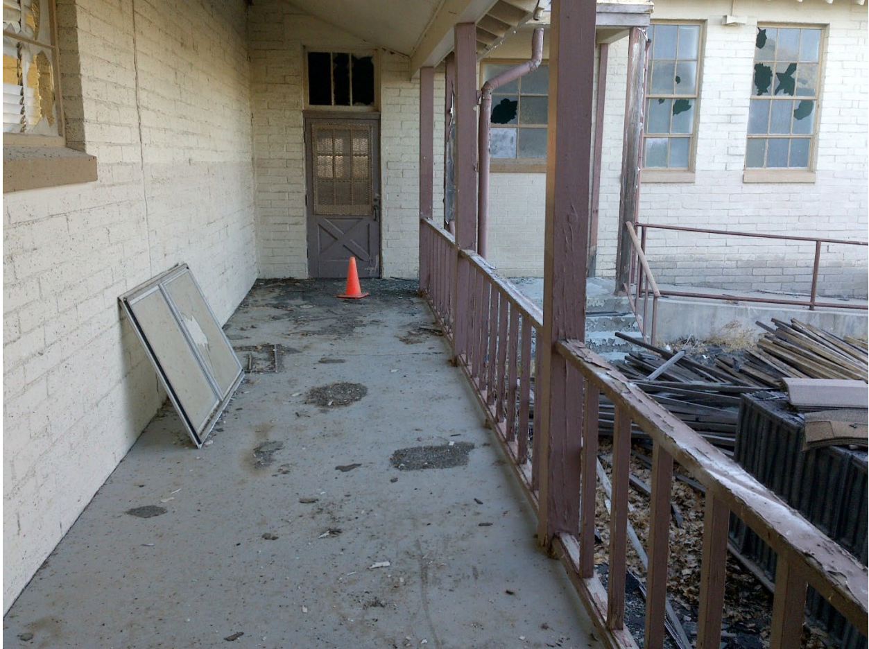
Figure 9. Courtyard walkway and railing visible in the background of the previous figure.
