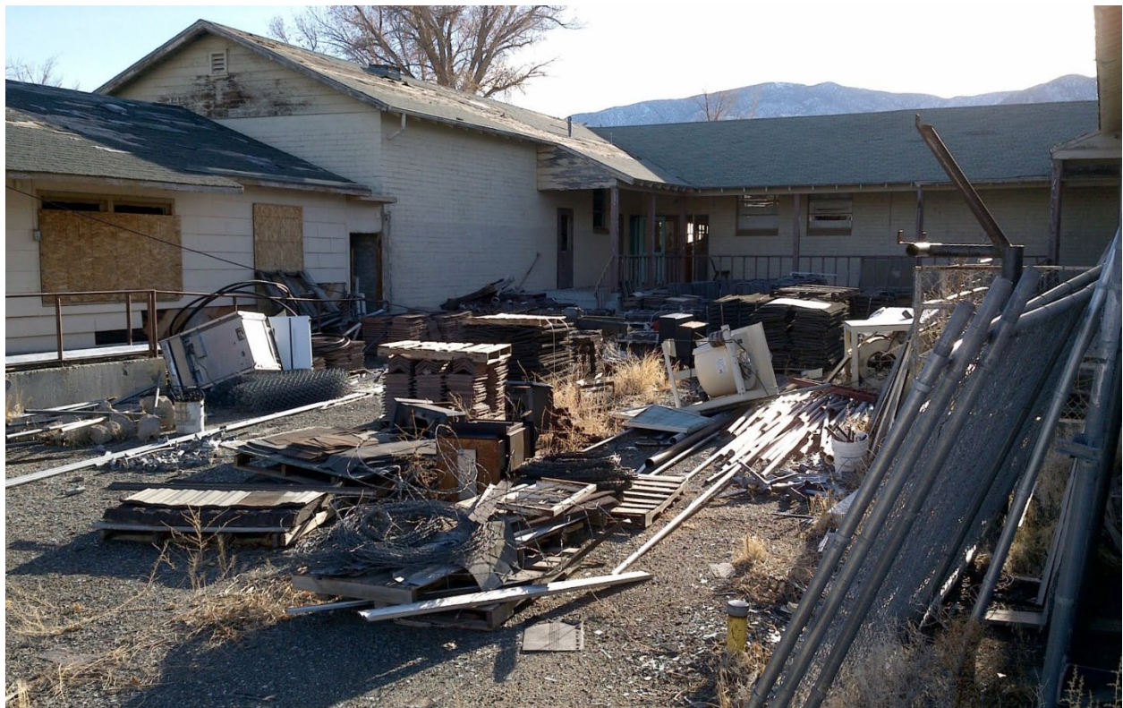
Figure 8. View looking southwest at the fenced courtyard area used for materials storage.
