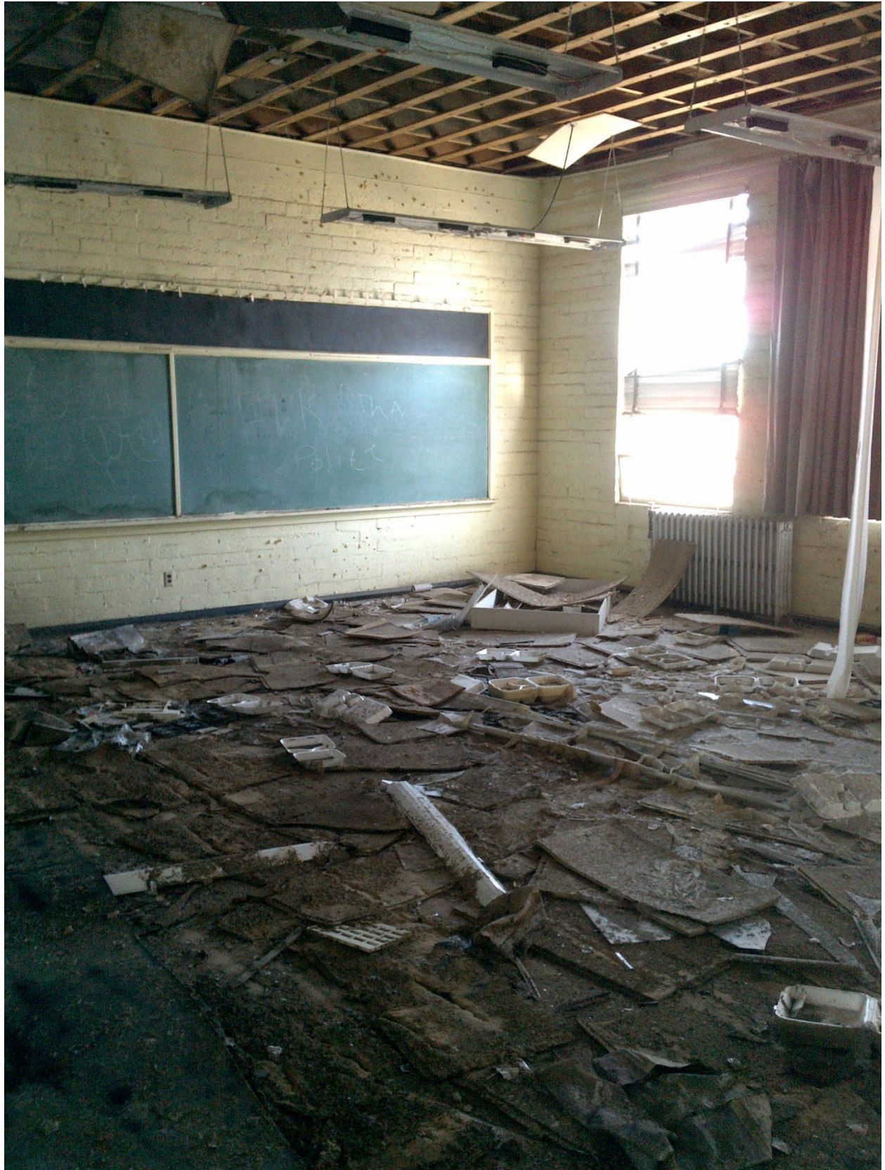
Figure 12. Abandoned classroom with ceiling debris and potential asbestos hazards.
