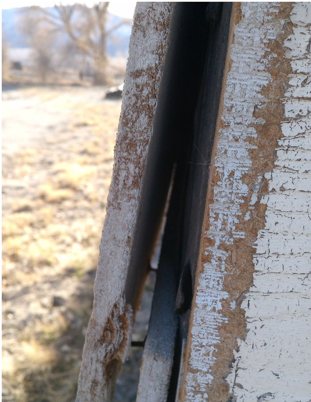
Figure 16. Potential lead paint hazard from flaking on the siding of the building in Figure 6
