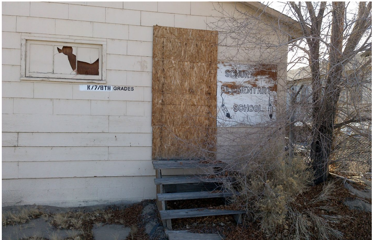
Figure 7. Boarded entrance to the structure in the previous figure (east side of the old school).
