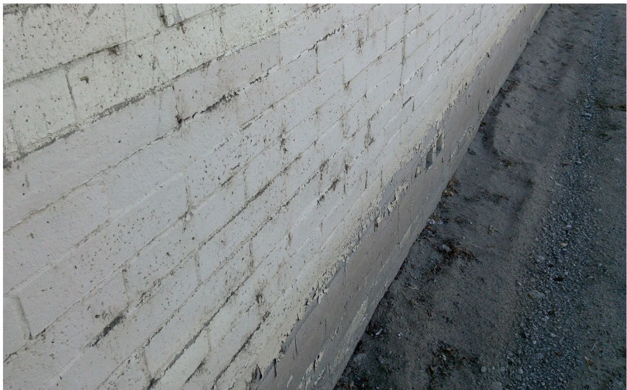
Figure 15. Potential lead paint hazard from flaking on the building's exterior brick walls.
