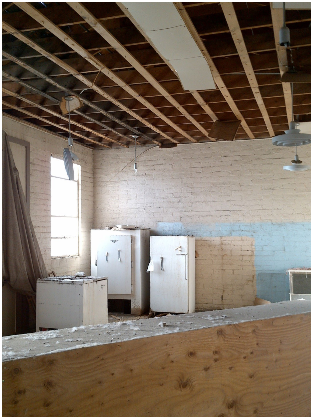
Figure 13. Additional room with ceiling failure and various abandoned appliances.
